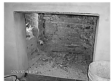
Badly Deteriorated Firebox
