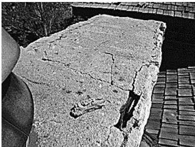
Damaged Chimney Cap
